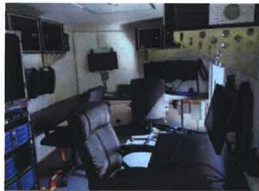
FIGURE 4-5: MOC TRAILER INTERIOR
